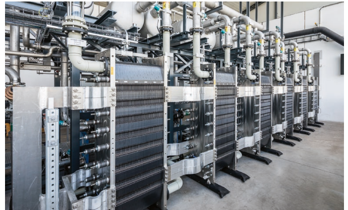
Image 03 – SIEMENS 6 MW Proton Exchange Membrane (PEM) electrolyzers (PRBX/ VOESTALPINE)
